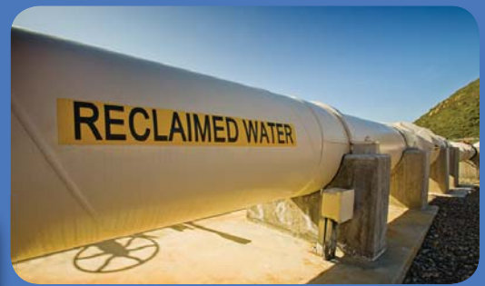
24-inch recycled water pipeline
