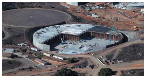
Aerial view of Twin Oaks Reservoir No. 2 under construction. Once complete, it will be buried to better blend with the environment.
